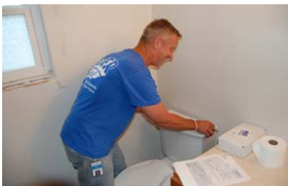
Replacing old water fixtures with new high-efficient models can generate valuable water conservation benefits.
